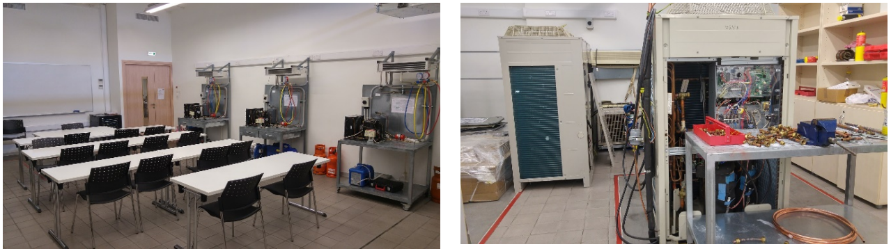
Figure 6: Refrigeration units (left) and VRV units (right).
